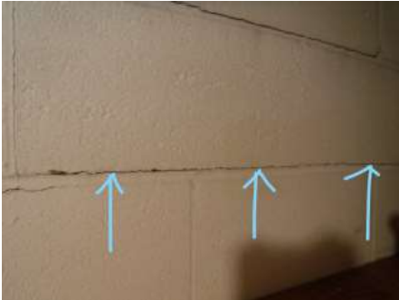
Minor horizontal crack in the front side basement wall
