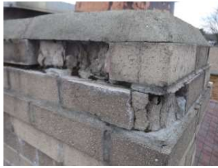
There are a few deteriorating/spalling bricks on the chimney
