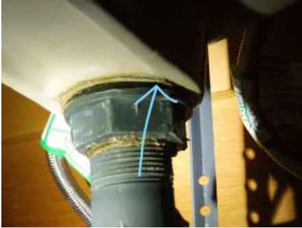
Main Bathroom - Sink drain is leaking at the sink bowl connection
