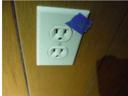
Some open grounds on receptacles in the basement
