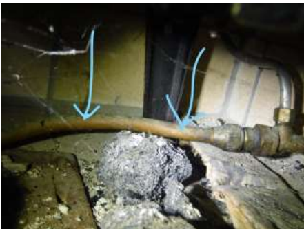
The copper gas line in the basement that is running to the fireplace are no longer used in today's installs per Gas Codes
