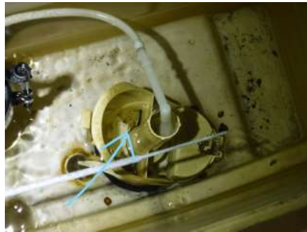
Basement Bathroom - The flapper inside the holding tank does not function properly, you have to hold down the flush handle the whole time until the toilet has fully flushed
