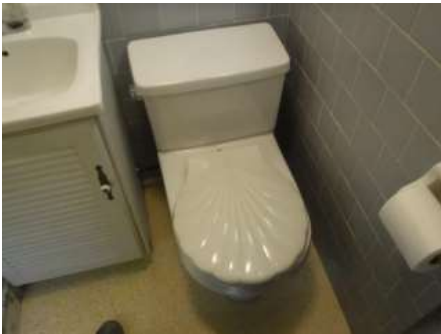
Master & Basement Bathroom - The toilets are loose from the floor
