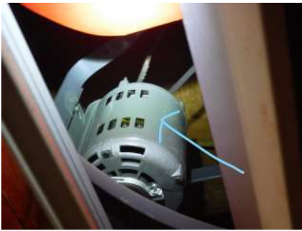
Whole house ceiling fan in hallway was inoperable, the motor appears to be seized
