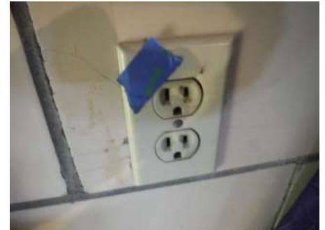
Open ground on a receptacle in the garage
