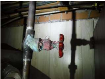
Corrosion on water tank shut-off valve from it previously leaking. No signs of any active leaking at time of inspection
