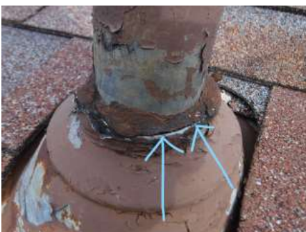
Mast Boot Flashing - Gaps/deteriorated sealant - Needs sealed
