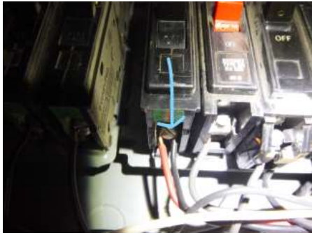
Double lug/tap breaker connection in main electric panel
