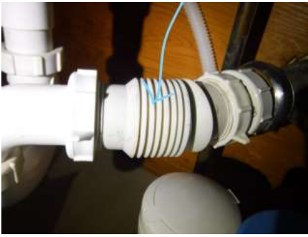
Section of the kitchen drain is an accordion style drain which are more prone to clogging
