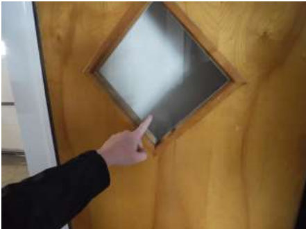
Garage man door is not fire rated
