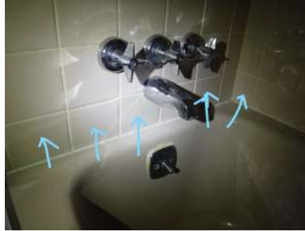
Main Bathroom - The lower row of tiles do not appear to be fully adhered to the wall surface
