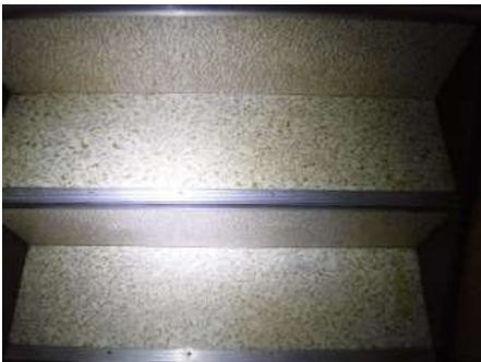
The linoleum/vinyl flooring on basement steps may contain asbestos
