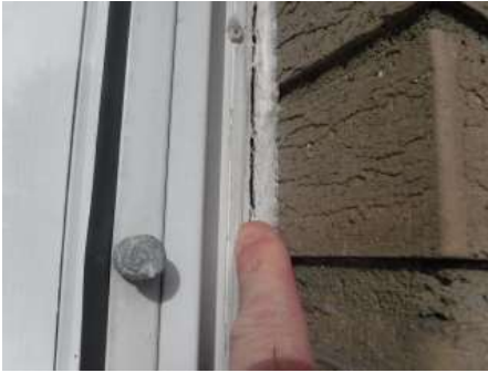
Gaps in the window flashing's - Needs re-caulked
