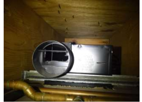
Basement Bathroom - The exhaust vent is improperly discharging above the drop ceiling
