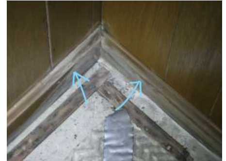
Signs of previous water wicking/staining at the bottom of the wall paneling/trim
