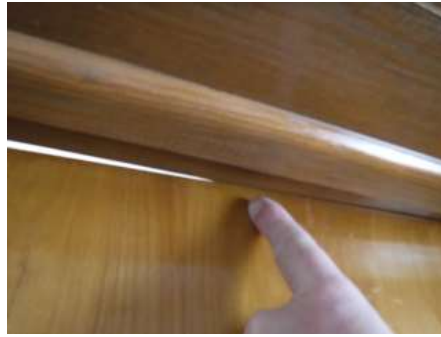
Master Bathroom - The door rub/sticks on the door frame
