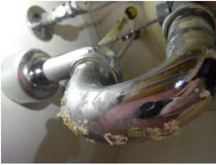
Master Bathroom - The sink drain is corroded
