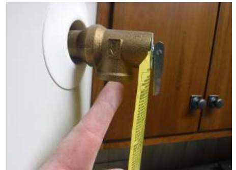
Missing down tube on the TPR valve
