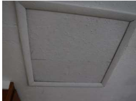
The plywood access panel to the attic on the garage ceiling is not fire rated
