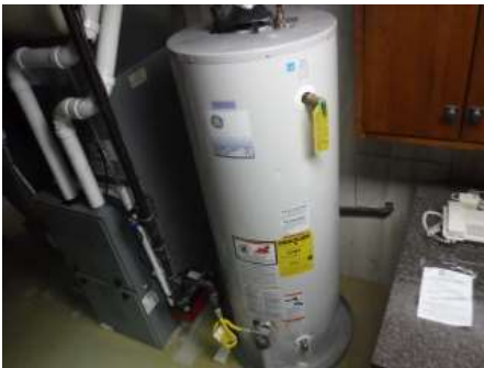
Water Tank Picture - Improper Draft/Back Drafting
