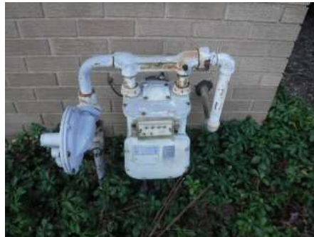
Gas Meter / Main Gas Shut-Off Valve Location
