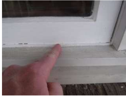
The two windows on the front bay window would not open, they appear to be painted shut
