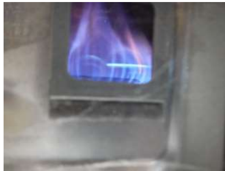
Water Tank Flames Picture
