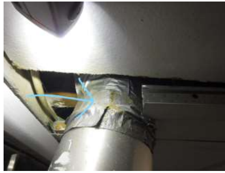
(Fire Hazard) - Improper use of duck tape on dryer exhaust ducting. Duck tape has the potential to catch on fire
