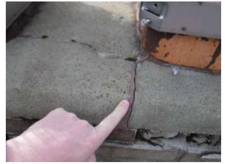
There are a few cracks in the topside of the chimney crown mortar
