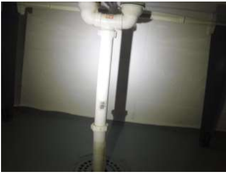
Utility sink drain is missing a trap to prevent sewer gas/smell from entering the home
