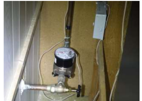
Water Meter / Main Water Shut-Off Valve Location
