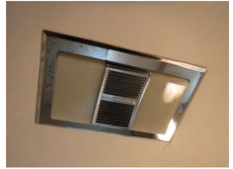
Main Bathroom - The bathroom exhaust fan is inoperable
